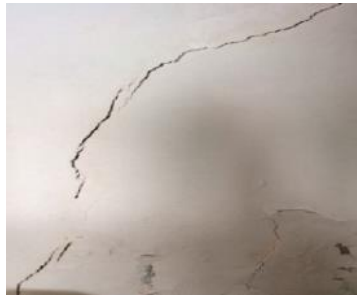
Existing Cracks on Wall
