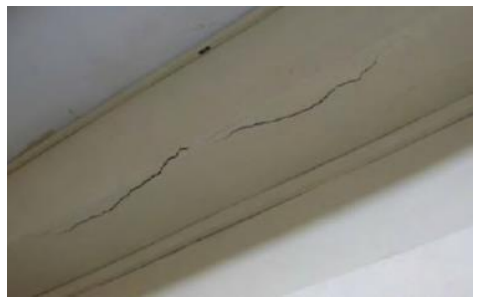
Cracks on beam
