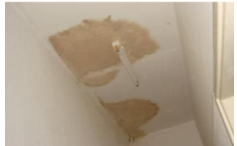
Water Seepage Stains
